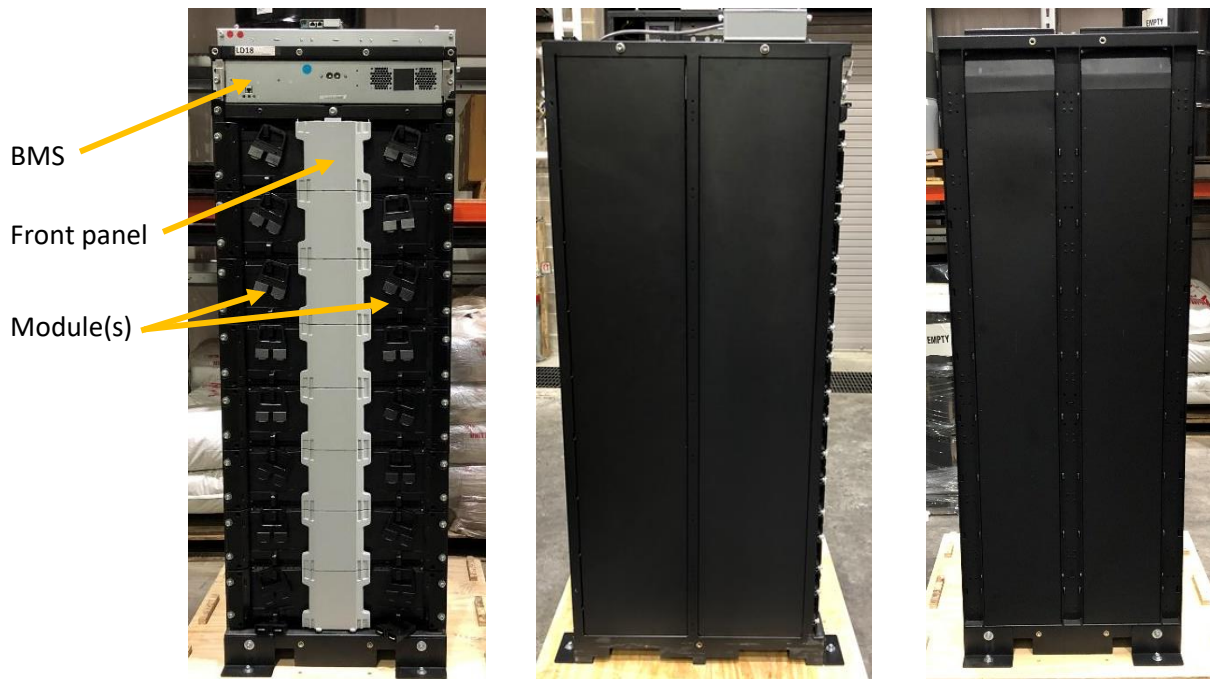
Figure 3-1: Photos of LFP rack; front (right), side (middle), and back (right).
